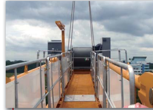
Large access to the hoisting winch for easy maintaining operation Every mechanism has one platform for the maintenance operation in order to work in safe conditions
